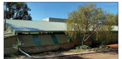
A new roof over the horseshoe bar with thanks to the Shire of Toodyay.
