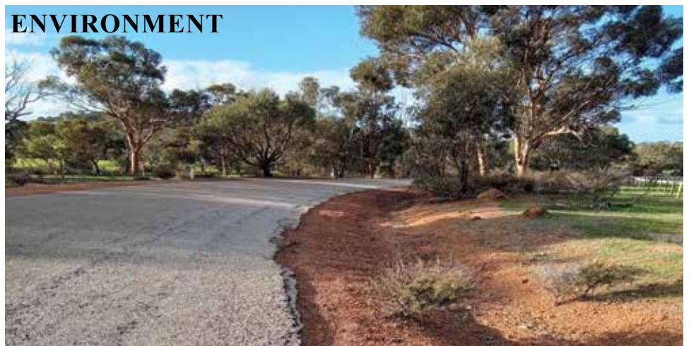
Crumbling road edges are especially dangerous on bends and crests. The above road is one of many in the Shire of Toodyay requiring maintenance work.
