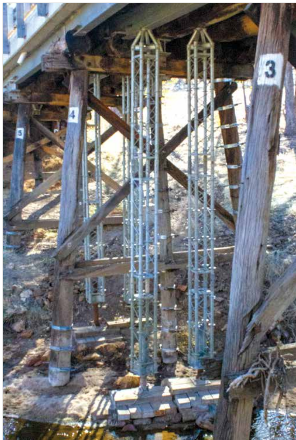
Underside of Slaughterhouse Bridge showing the temporary props and metal straps around the weathered timber pylons.
