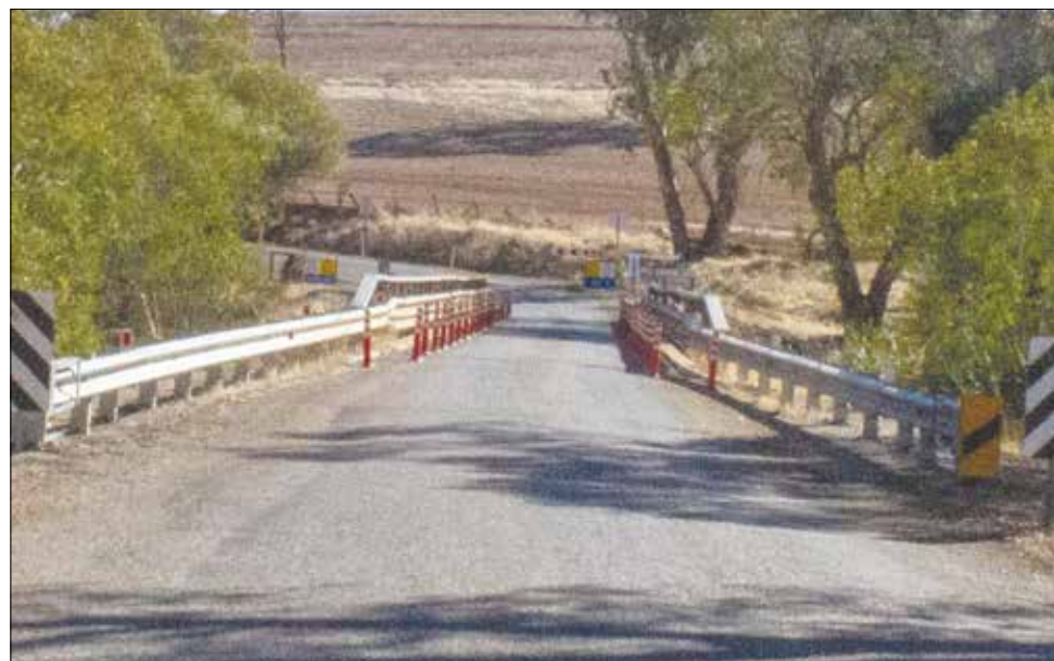
Slaughterhouse Bridge showing some of the traffic control measures currently in place.
