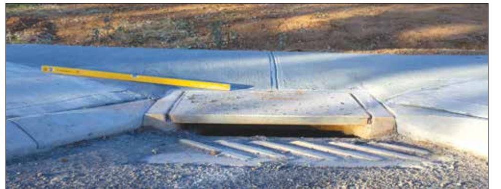
Toodyay Street footpath slopes down onto a stormwater drain lid.
