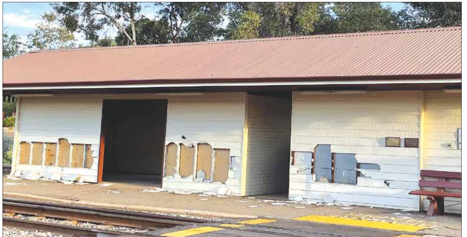
More vandalism at Toodyay railway station.
