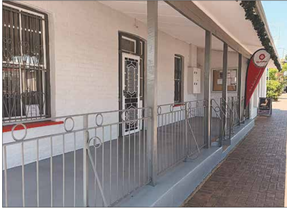
The newly painted front of the St John Sub Centre Administration building on Stirling Terrace.
