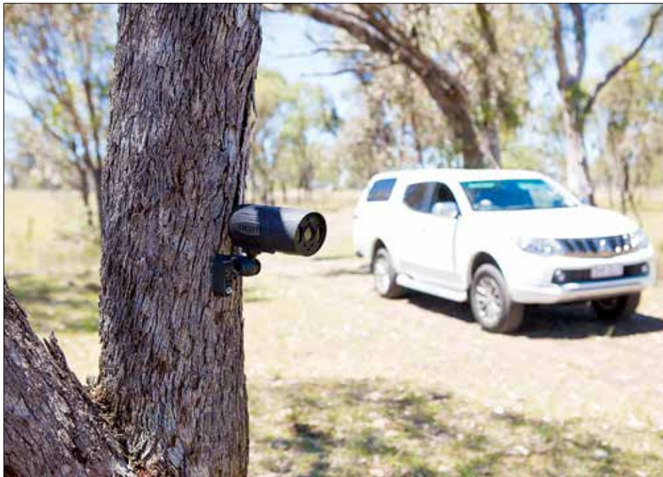
CCTV cameras are a good deterrent against thieves.
