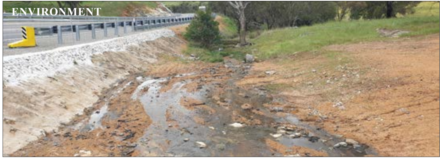
Run-off from roadworks on Toodyay Road near Coorinja Winery pollutes Harper Brook which flows into the Avon River near Extracts Weir.
