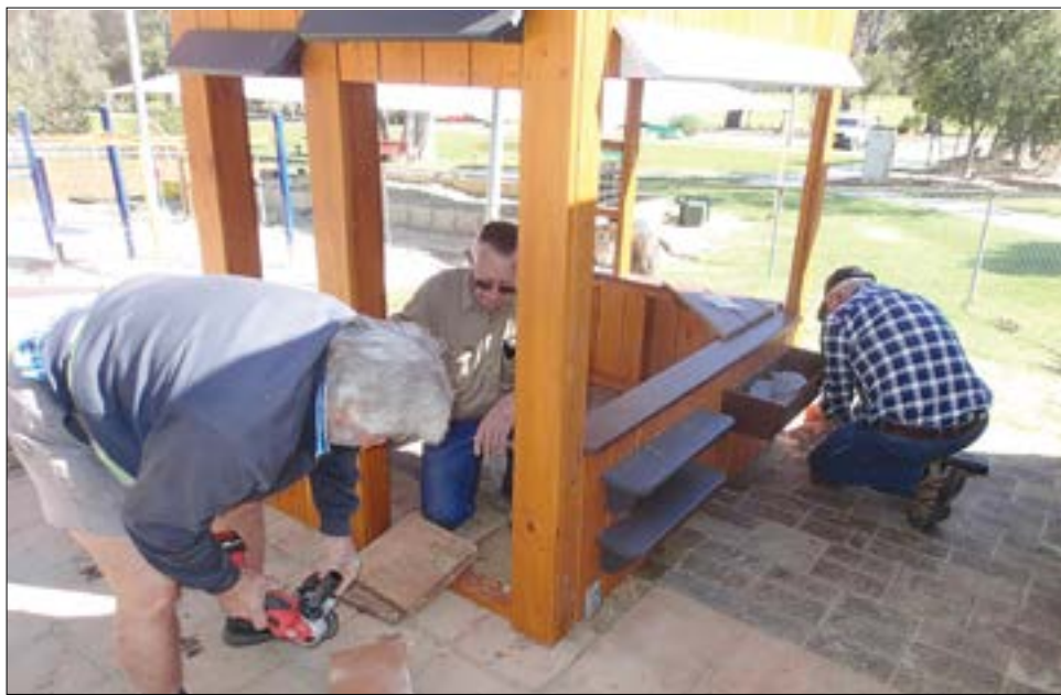
Moondyne Men hard at work on cubbyhouse construction for Toodyay District High School students
