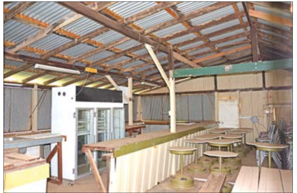
Rafter support beams sag under the weight of the metal roof.
