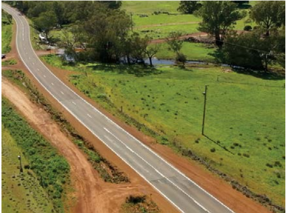
Construction is underway on a short section of Toodyay Road adjacent to Coorinja Winery
