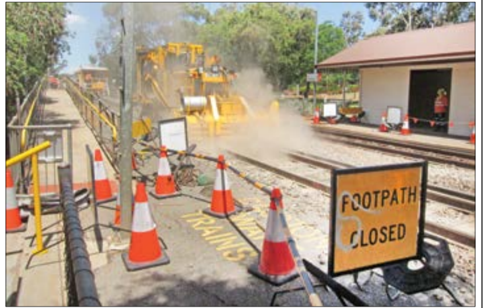
Toodyay Station pedestrian crossing was closed three days for bitumen repairs last month.
