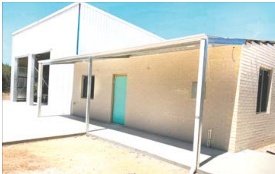
New Julimar Fire Station construction complete and now being fitted out for action.
