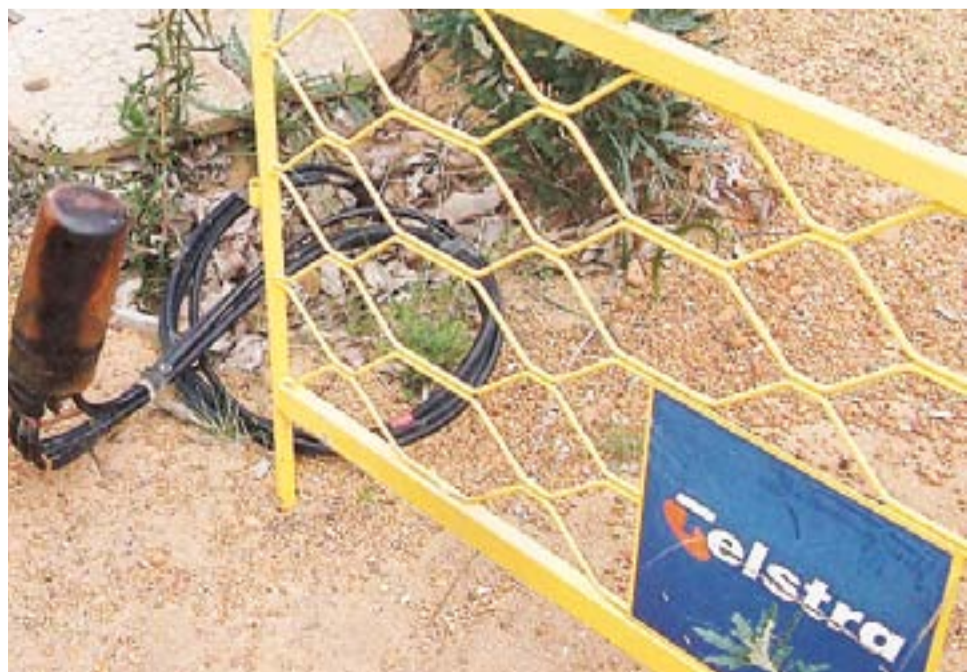
Broken Telstra cable box at corner of Blackbutt Drive and McKnoe Drive has not been fixed for two years
